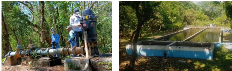
Image 2. Guluchapa WSS infrastructure
